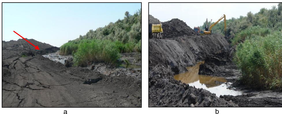
Fig. 3 Phenomena of slag heap collapse in Mălina Creek: a - riverbed blockage; b - works to restore the riverbed (Bălan, 2010).
